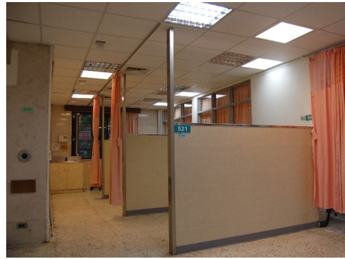
Figure 1 Room with LED lamps.
